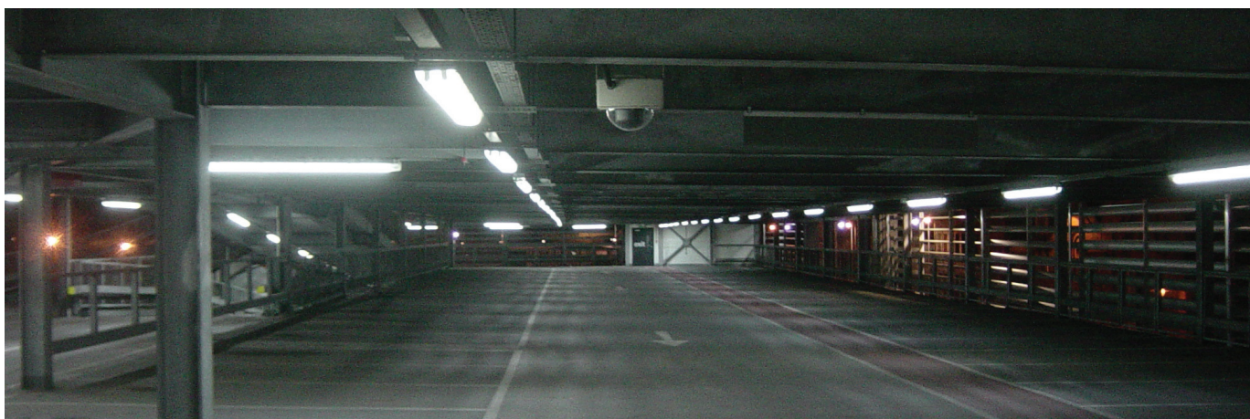
System with all lights activated
